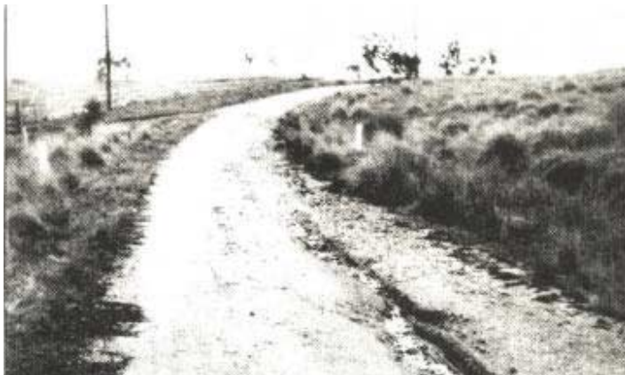
Plate 8 – Road surface erosion – Shuter Avenue
