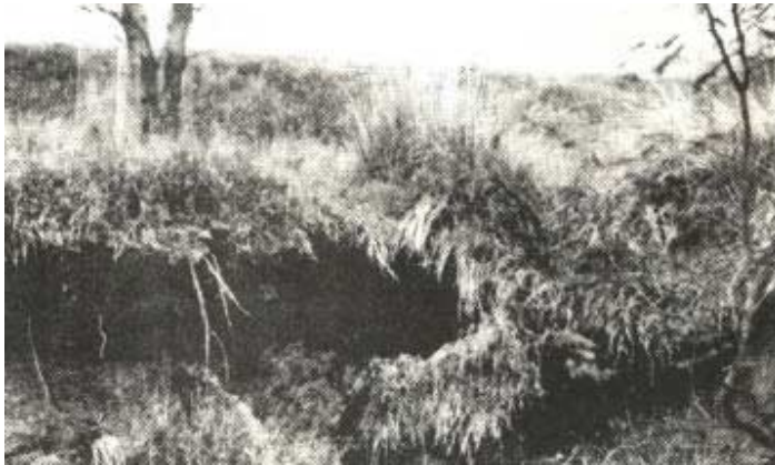
Plate 10 – The top of a 5 m deep bully head on Lot 127 is below the well grassed dam bank
