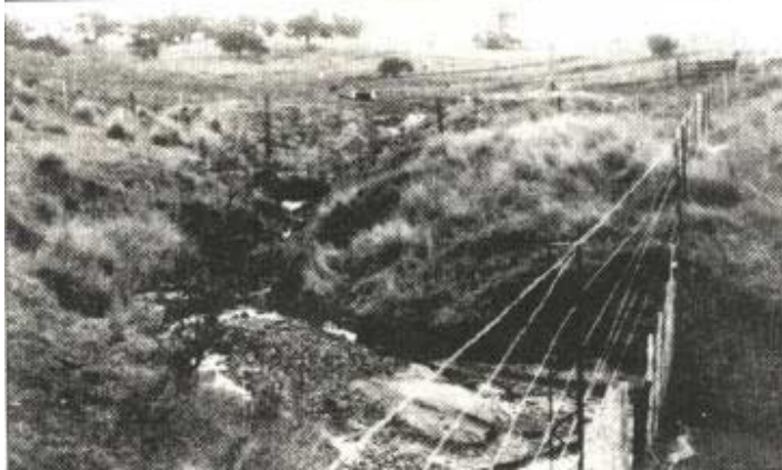
Plate 7 – Sediment in the gully floor from a failed dam. This will reduce the capacity of the dam further down the drainage line
