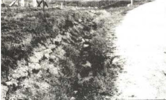
Plate 9 – Table drain erosion – Shuter Avenue
