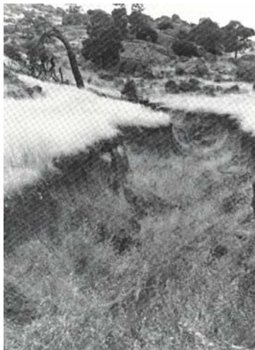
Increased run-off from the cleared, rocky hills saturates and erodes the deep sandy soils.
