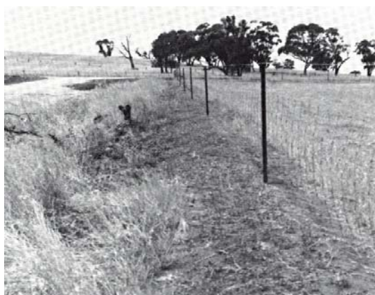
Increased run-off from adjacent hills does cause severe gully erosion on the upper slopes in soils that have a high slaking tendency.
